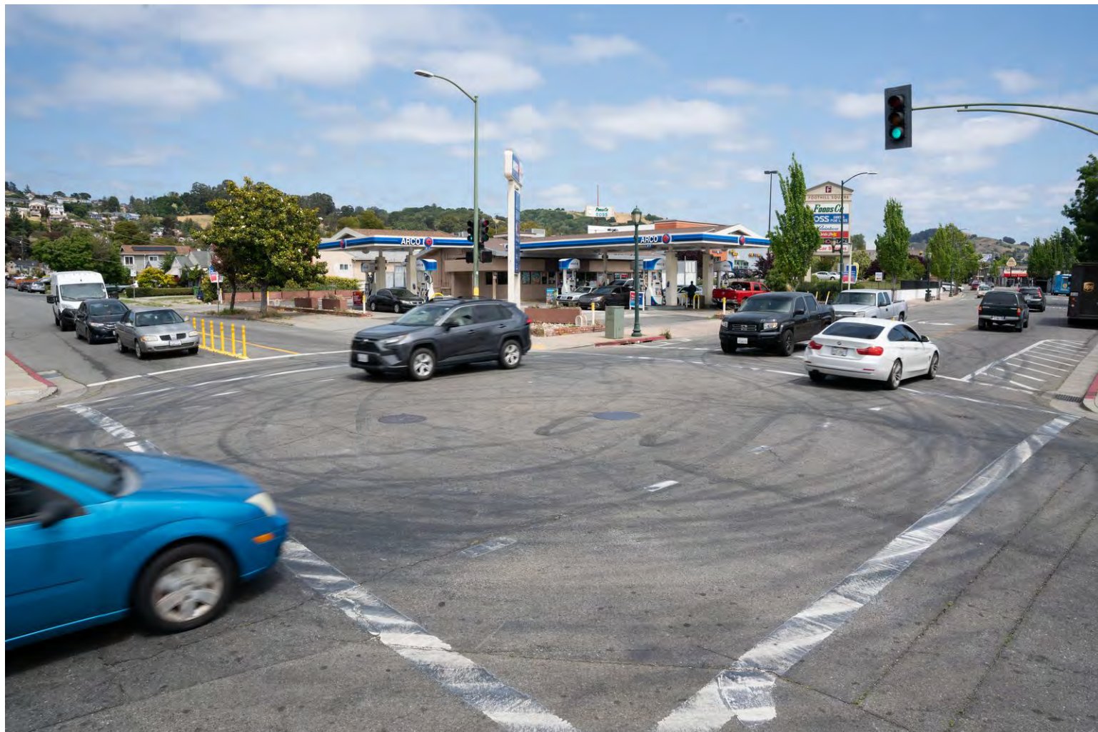
The intersection of 106th Avenue and MacArthur Boulevard was ranked second for the number of sideshows that happened there among all city intersections in 2022. Credit: Florence Middleton
